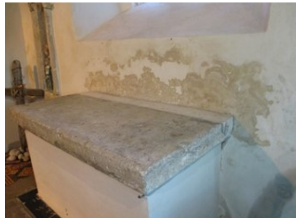
Water damage behind the altar, which has been cemented to the wall
